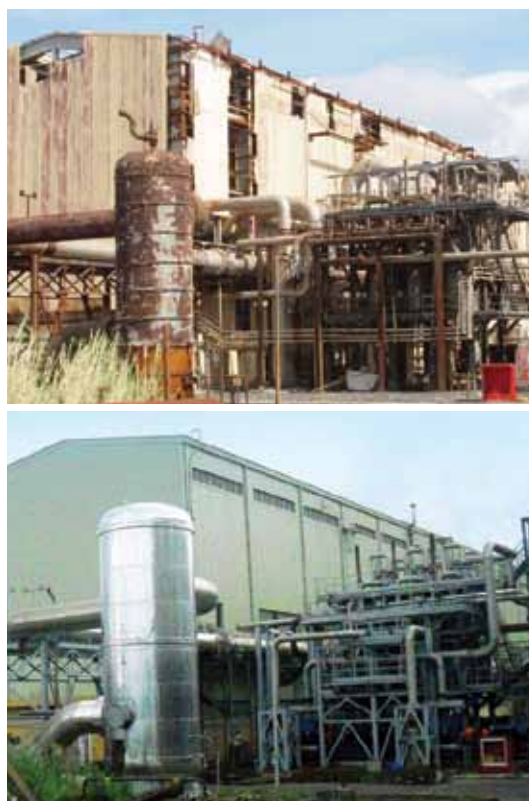
Non-operational Bacman was acquired on an "as is, where is" basis. Despite the setbacks, we are optimistic that it will generate strong revenues and cash flow once fully operational. Photo shows the Palayan power plant before and after refurbishment.
